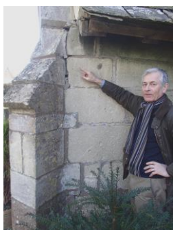
Jonathan points out one of the cracks on the porch
